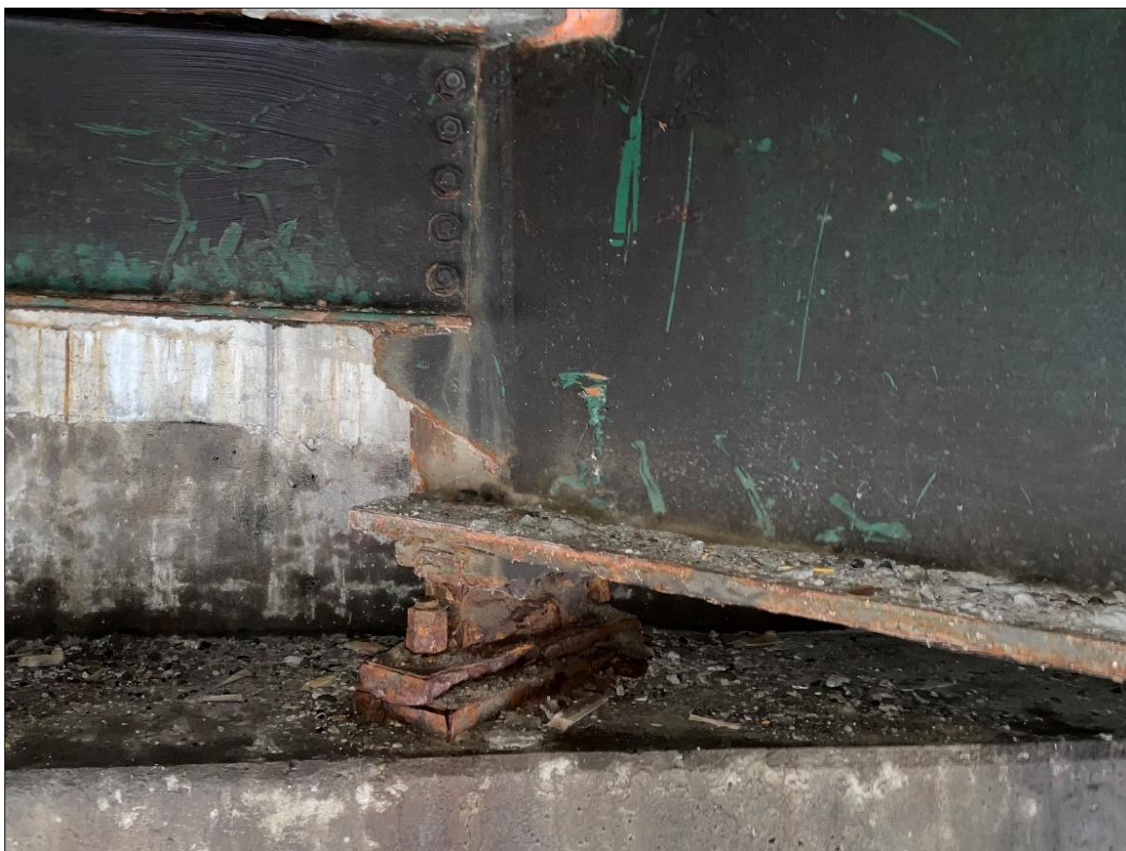
Bridge 25S Southern Abutment Typical Bearing Condition
