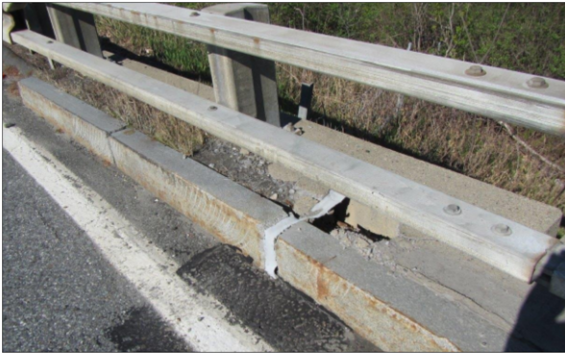
Bridge 27S Curb Deterioration at Bridge End
